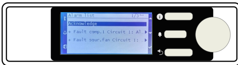
Figure no. 5 Alarm list
